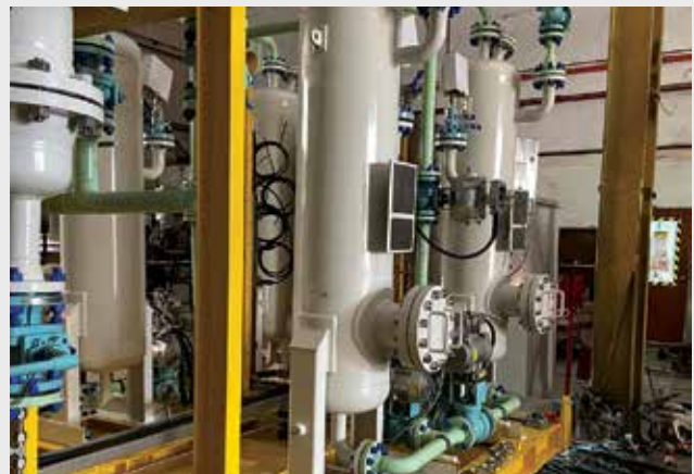
The state-of-the-art 2 X 100% air dryer skid installed and commissioned to achieve a demand of -40degC dew point as stated in ISO 8573 standard for instrument air quality, in Sarawak Water.
