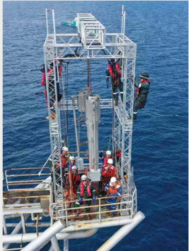
A specialized offshore team executes a flare tip replacement using rope access technique with precision and on a remote offshore platform, in Peninsula Malaysia Waters.
